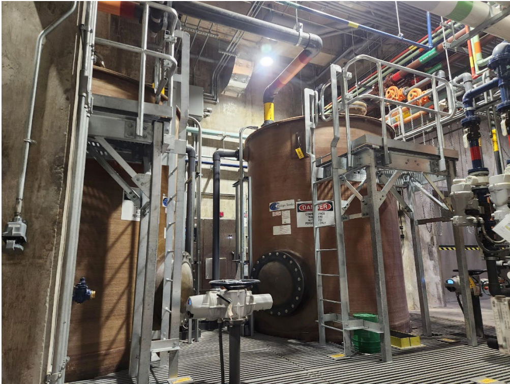
LADDERS AND PLATFORMS IN POLYMER AREA
