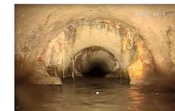
Picture above: Root intrusion into pipe indicates likely infiltration of clear water and can block sewer flow. NEW Water Television Program
